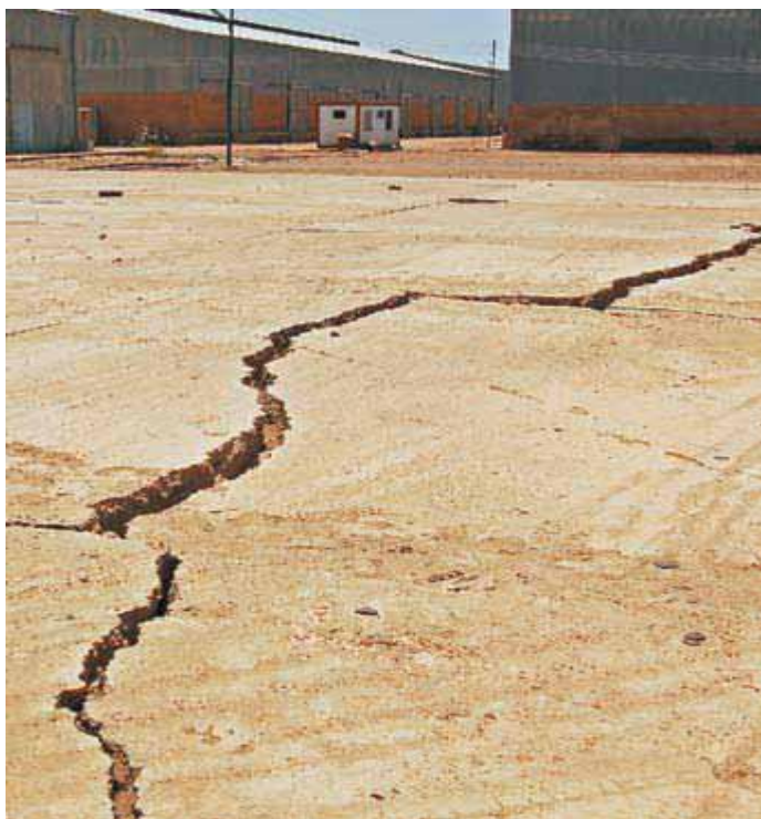
Plate (2) This cement-lined pit in Hasahesa – where an obsolete pesticide stockpile has been buried – has cracked, releasing a strong stench and exposing groundwater to a high risk of
